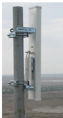
Fig. 10. Access point of the center of a wireless communication network of NSSM
