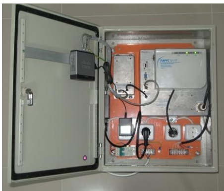
Fig. 8. Field unit of the NSSM system for land installation
